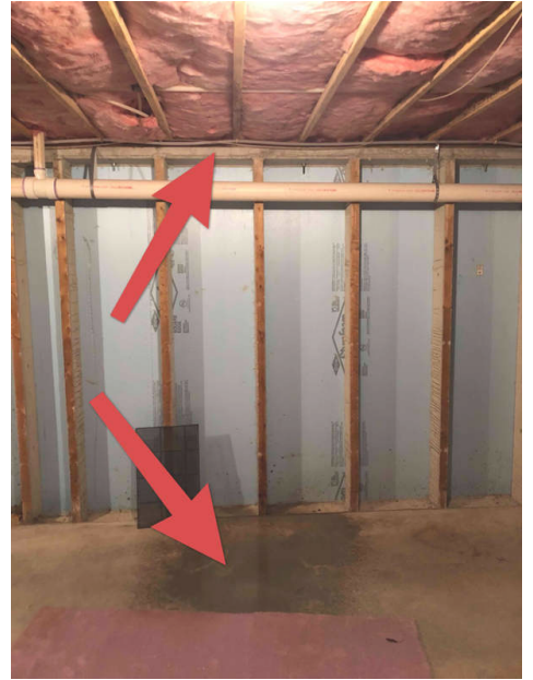
Evidence of leak
