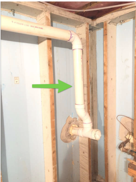
main soil line
